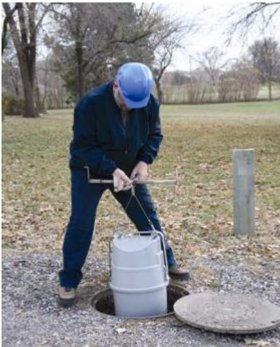
Below grade sampler installation
